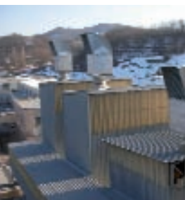
← (photo 2) Bulk loading units chimneys silencers ARQUATA SCRIVIA (ITALY)
