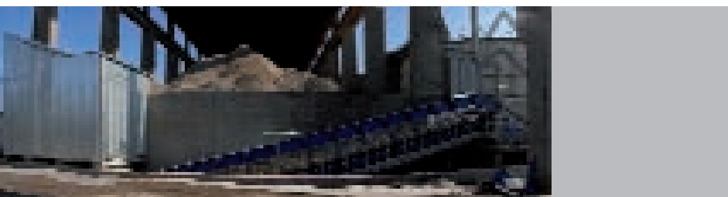
↑ (photo 1) Raw material conveyor belt ARQUATA SCRIVIA (ITALY)
